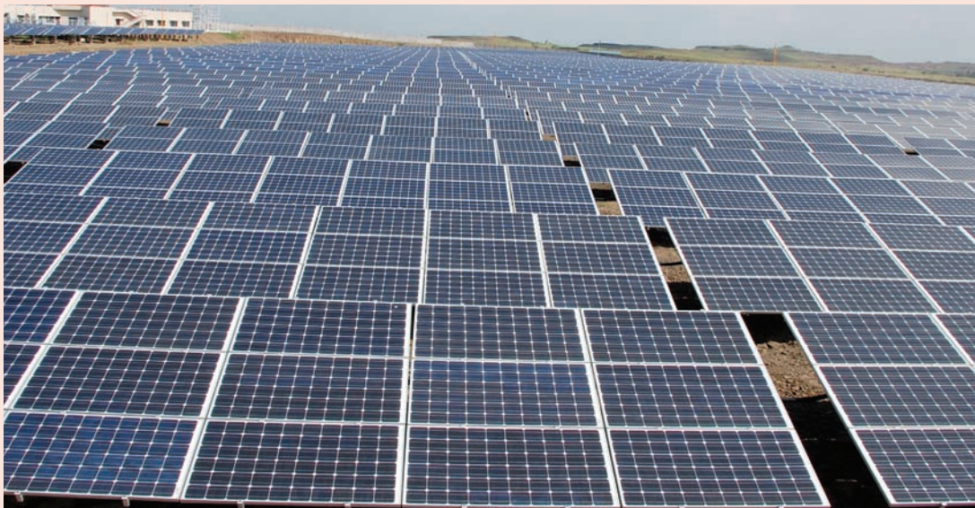
Itnal Solar Power Project
